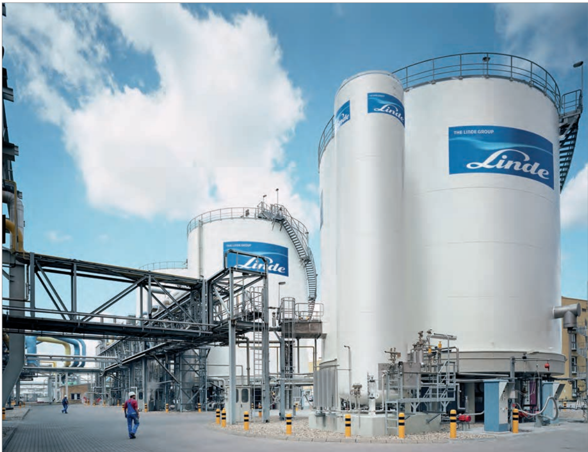
Fig. 48: In addition to oxygen, nitrogen and argon, the air separation unit in Leuna also produces crude neon, crude krypton/crude xenon and helium, photo: Linde AG (with kind permission).
