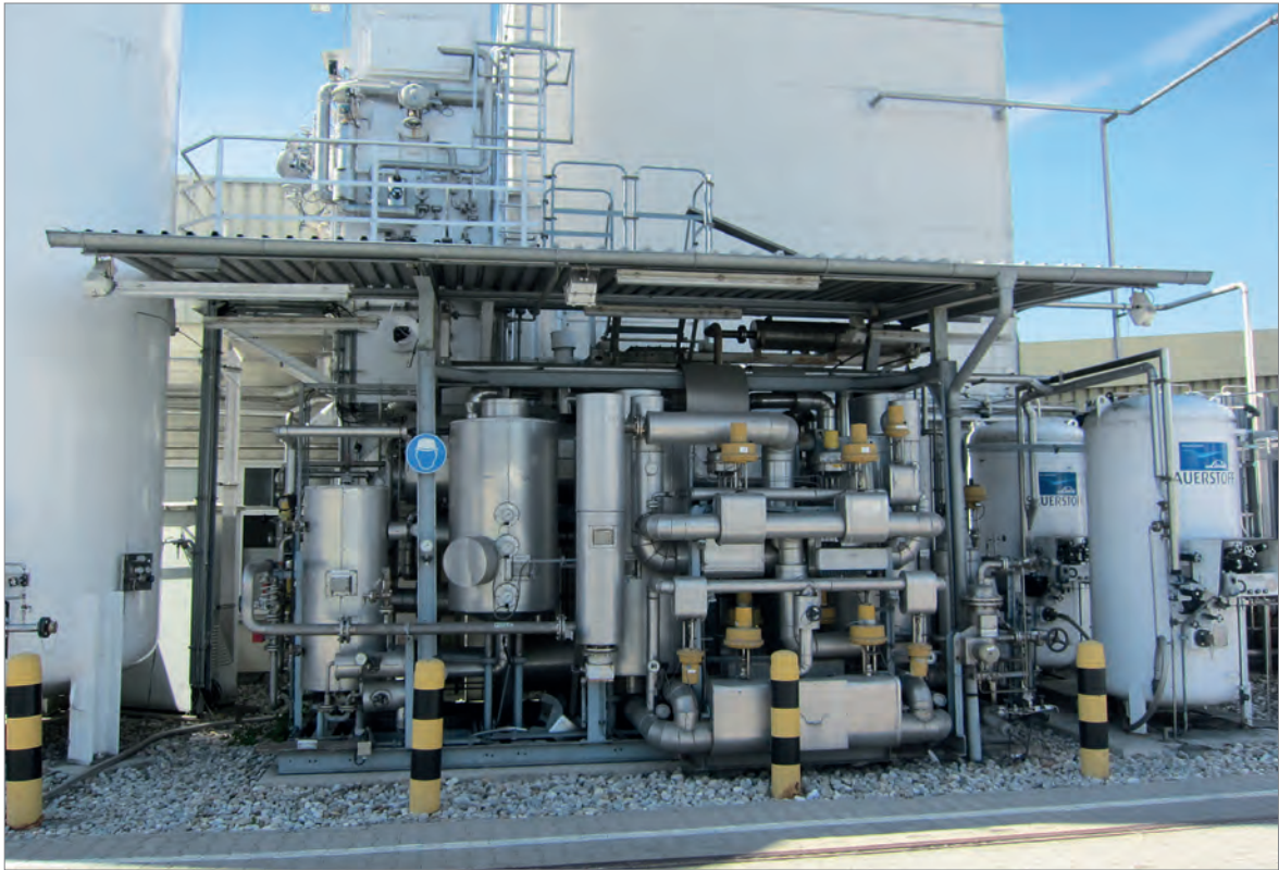
Fig. 51: View of part of the crude krypton and crude xenon purification plant at Linde AG's Unterschleißheim plant, photo: BGR.
