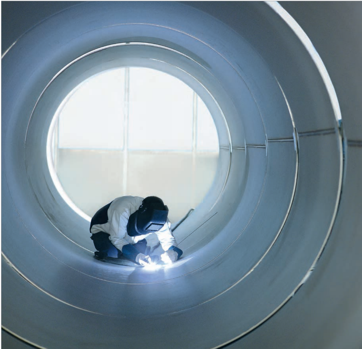
Fig. 15: Stainless steel is usually welded using the tungsten inert gas method in an inert gas atmosphere of argon or, more rarely, helium, photo: Linde AG (with kind permission).
